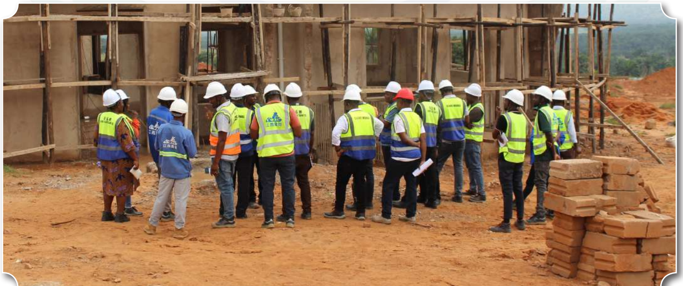
Members of the MUHAS HEET PIU team inspects the progress of construction works at the Kigoma Campus.
