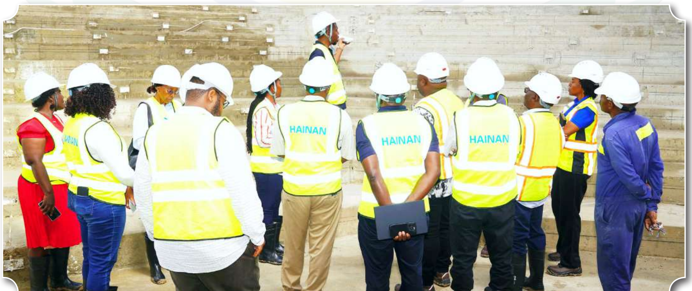
Members of the MUHAS HEET Implementation Unit inspecting the progress of the Lecture Hall Theatres construction at the Mloganzila Campus.
