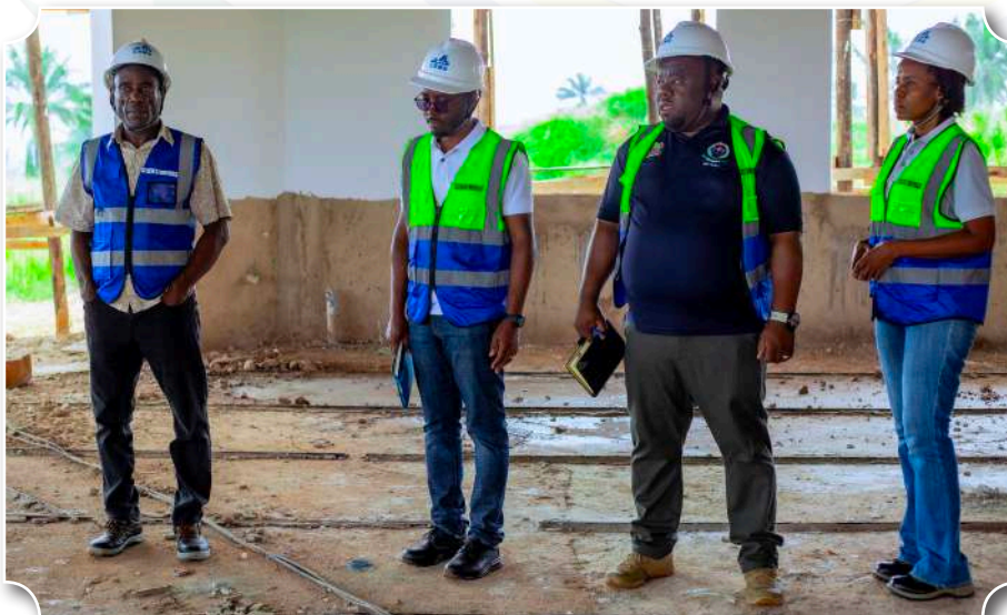
The Vice-Chancellor, together with the MUHAS HEET Project Deputy Coordinator, the Project Manager, and the Head of the Communication and Marketing Unit, inspects the ongoing construction of the new MUHAS Kigoma Campus
